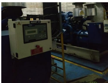
Gambar 10. Control Panel Genset
